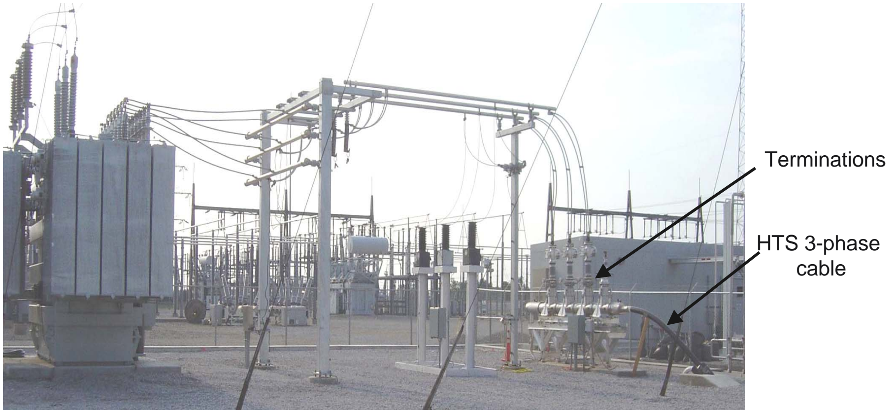
Bixby substation, AEP, Columbus OH 13.8 kV, 2400 A 200 m cable system by Ultera (Southwire/nkt cables) In-grid operation since July 2006
