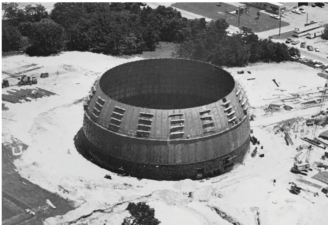
The High Flux Beam Reactor (HFBR) containment vessel under construction at Brookhaven National Lab in June 1962. The HFBR operated for more than 30 years before being shut down in 1999. Credit: Courtesy of Brookhaven National Laboratory
