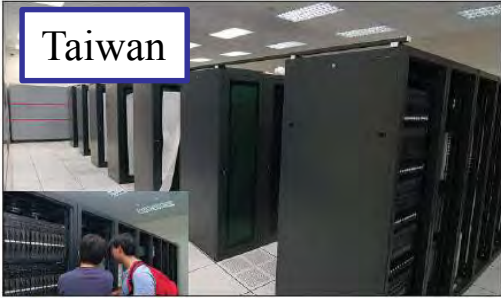
The data centre at the ASGC with 400 KSI2K computing capacity.
